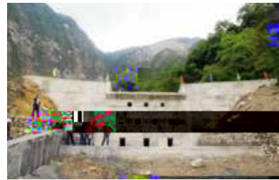
Engineering mitigation for debris flow hazard (check dam)
